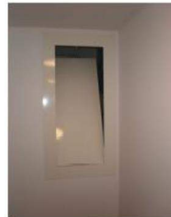
Figure 4 – Smoke Shaft Ventilator
